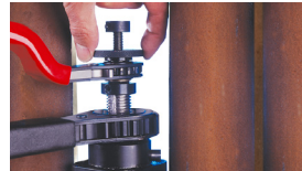
Tube overlay is efficiently removed from the tube O.D. and the tube end simultaneously beveled in preparation for welding.
