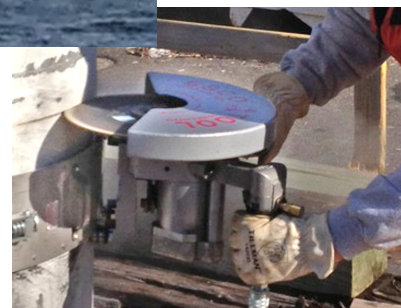
Scoring concrete pilings for height trimming. Concrete Cut-Off Blades are available in Diameters of up to 14".
